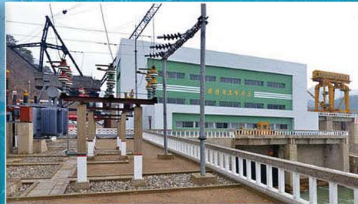
Huichon Power Station No. 8
