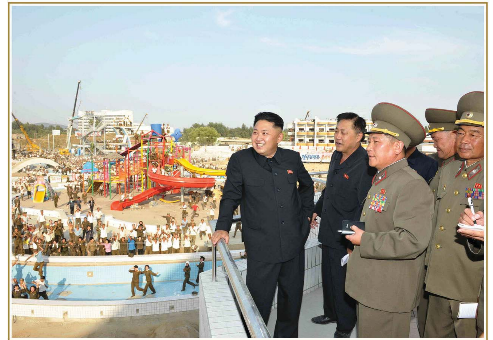
Kim Jong Un inspects the construction site of the Munsu Water Park [September Juche 102 (2013)]
