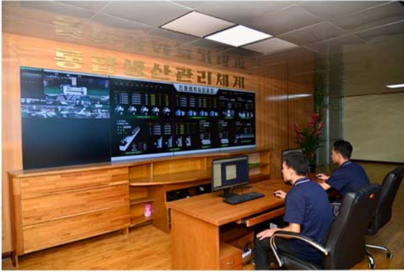
The integrated control room.
