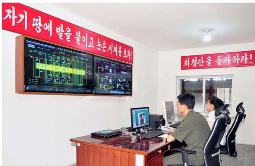
The control room for anthracite gasification and high-temperature air combustion calcination processes.
