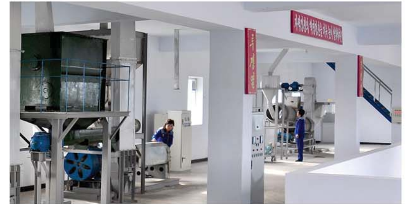
The interior of the feed processing workshop.
