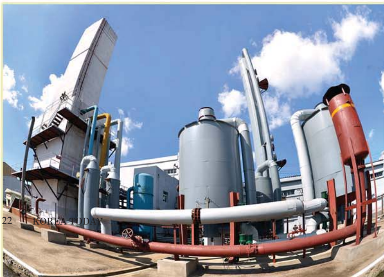
A view of oxygen plant workshop No. 1.
