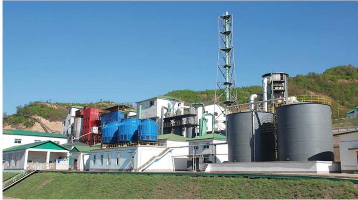
Sulfuric acid production
