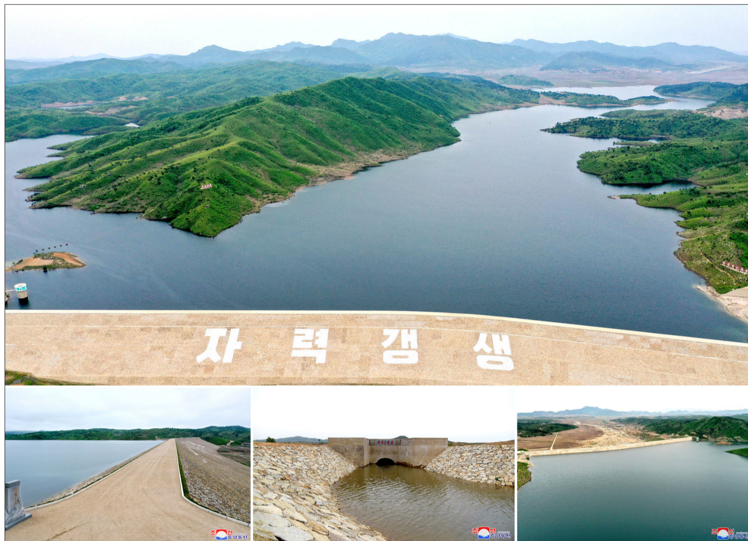
Dam on Lake Pongchon and other structures of the waterway in South Hwanghae Province.
