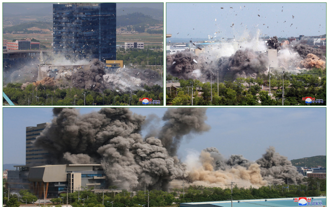
The four-storey north-south joint liaison office located in the Kaesong Industrial Park is completely pulled down at 14:50 on Tuesday.
