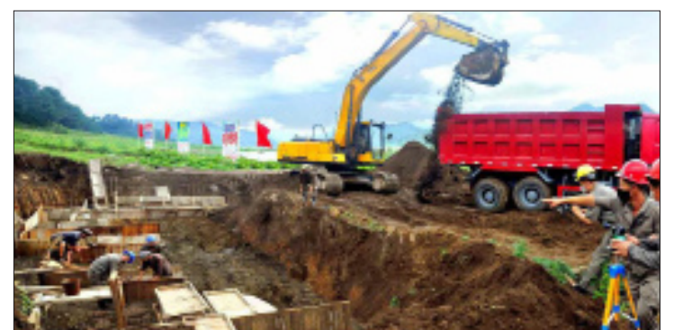
A reconstruction work is under way in flood-stricken Ichon County, Kangwon Province.
