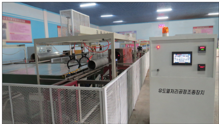
Induction heat treatment process control system developed by the power electronic technology institute under the State Academy of Sciences.
