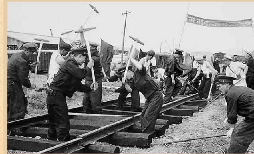
Railway workers laid in only 75 days 80km of standard-gauge railway lines between Haeju and Hasong.
