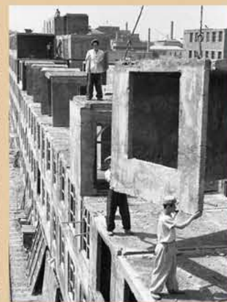
The construction workers of Pyongyang built over 20 000 flats with the materials and funds for 7 000 flats in one year, thus creating the Pyongyang speed during the great Chollima upsurge.
