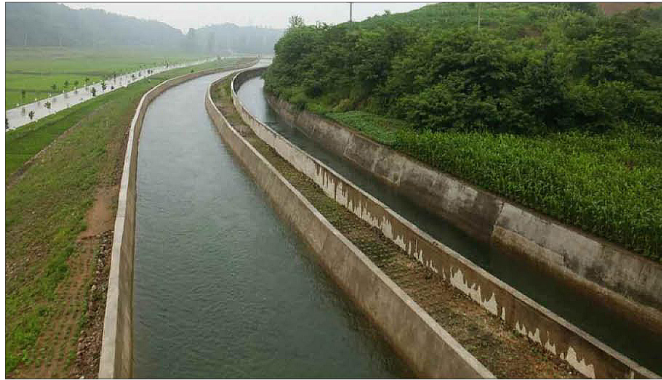
A part of the River Chongchon-Phyongnam irrigation waterway. RODONG SINMUN
