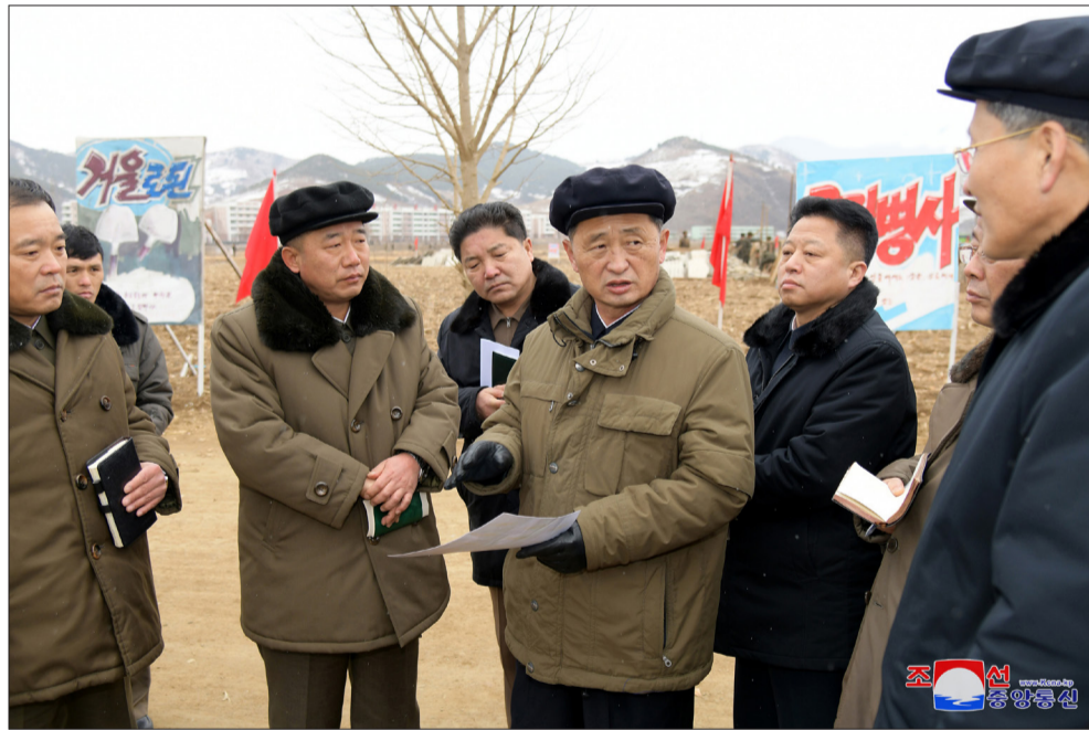
Premier Kim Tok Hun (fourth from right) inspects the construction site of a regional industry factory in Yonhan County.
